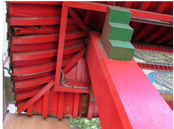
Figure 4.48 Deteriorated timber rafter and damaged plywood soffit.
