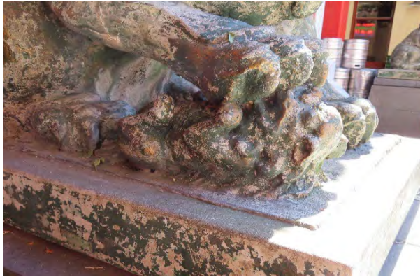
Figure 4.51 Poor condition of the painted concrete lion.
