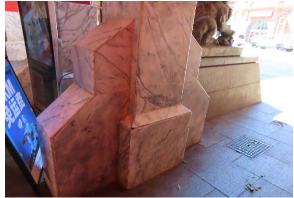
Figure 4.52 Chipped marble plinth.
