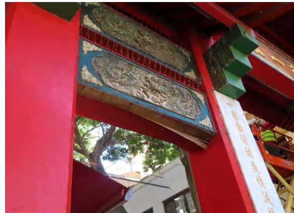
Figure 4.33 Peeling plyboard beneath decorative panel D.
