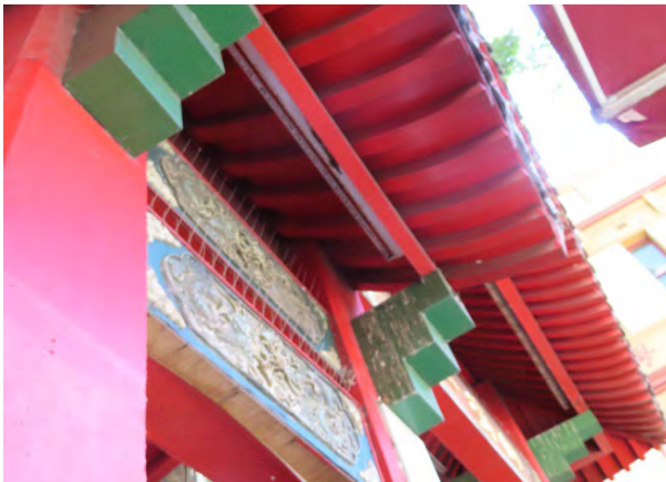
Figure 4.47 Delaminating plywood on the lower decorative panel D.
